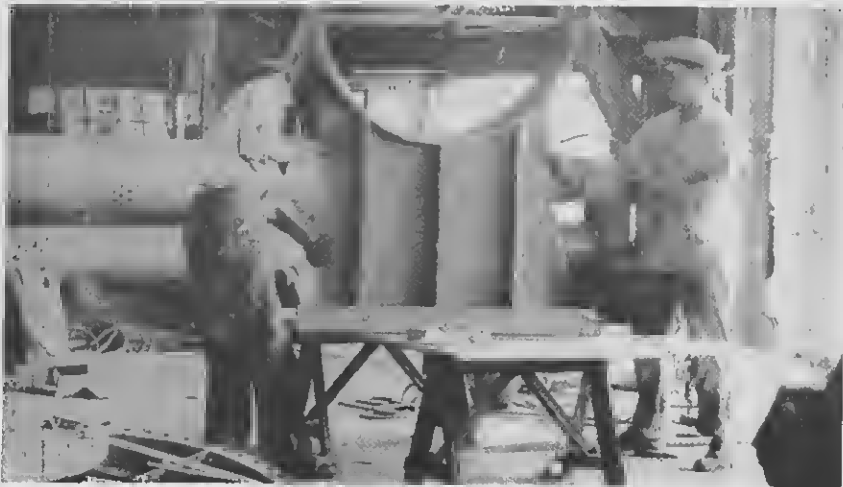
Boiler shop (5). Two boilermakers study the problem of repairing a saddle for an exchanger from one of the process units. Note plate roll in background which is used to curve boiler and tank plate.
